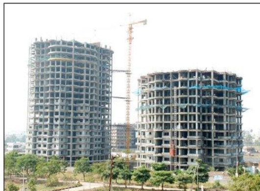
Ongoing construction activity at Yatra's Saket residential project in Hyderabad – the project is expected to be completed by March 2010
